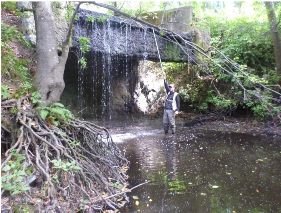
Figure 24: Downstream extent of the undermined Jewel Lake Spillway.
