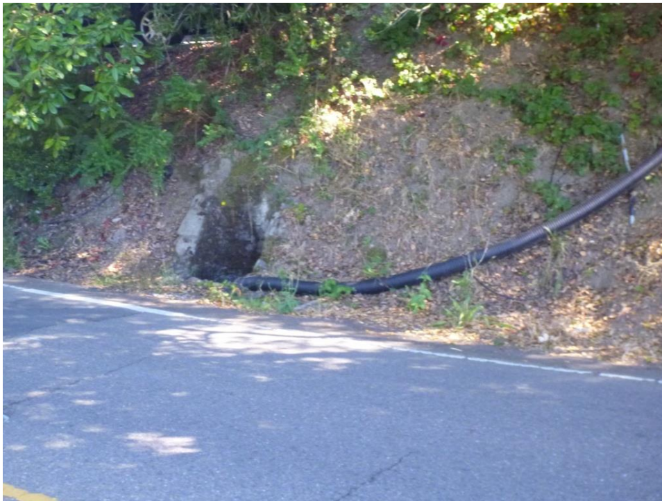
Figure 28: Plastic pipe transporting runoff from a residential gutter directly into the stormwater drainage system along Wildcat Canyon Road.
